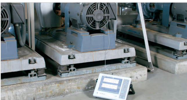
Vibration measurement in a plant using the CF-7200A and the NP Series Accelerometer
